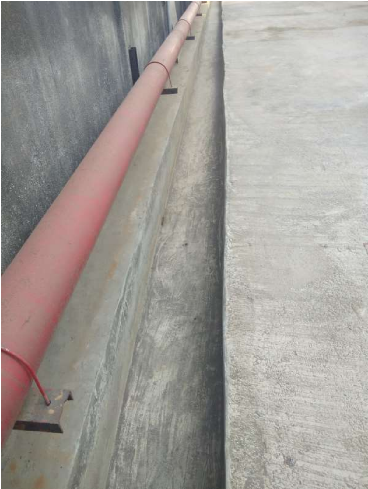
Anuh Pharma Ltd, Tarapur Storm Water separate Drainage
